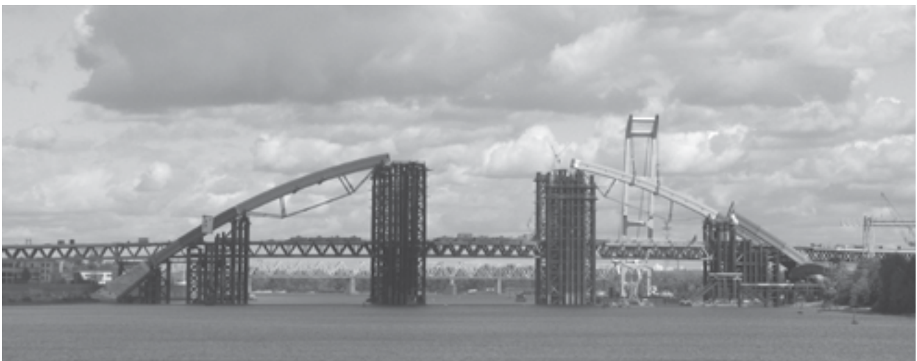
The construction of the Podil-Voskresensky bridge to unite right and left banks of Kyiv city (the subway extension from the right bank to Troieshchyna and Raiduzhny residential areas on the left bank of the Dnipro River) has been already lasting for 13 years
